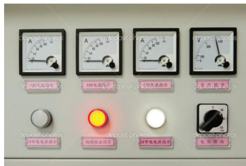
Figure 7.16 ▲ Measuring electricity in power houses and electrical generators
