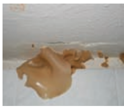
fungi on walls
